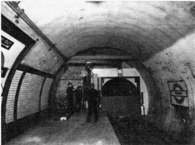
Manual Floodgate inserts from the 1930s using metal plates instead of timber.
